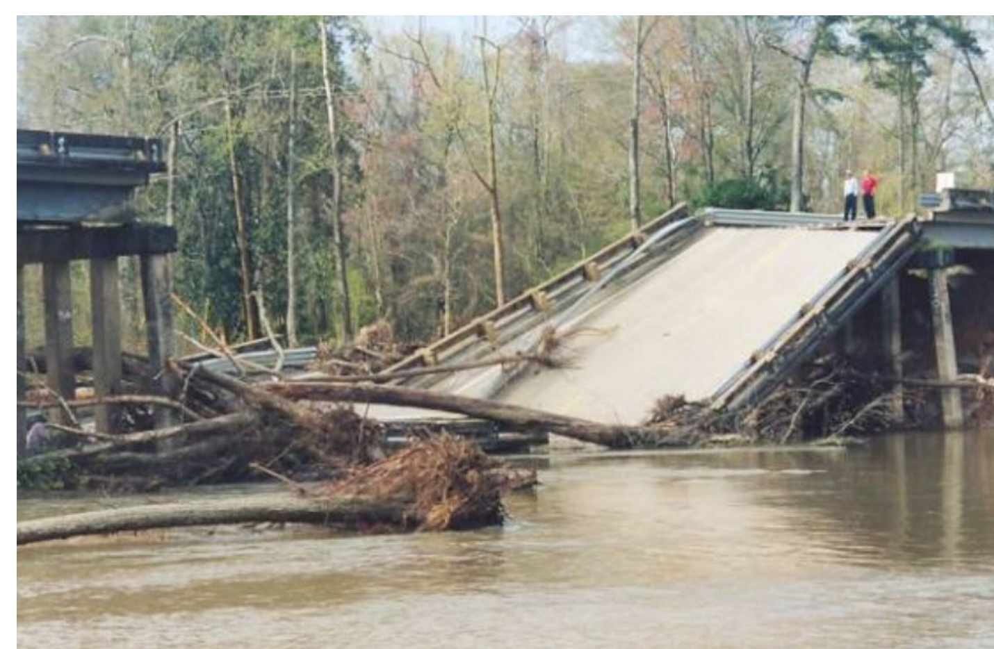
Figure 1: Bridge pier failure due to scour (FHWA HEC-09)
