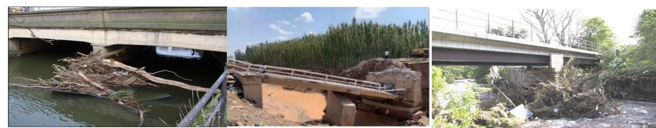
Figure 1. Debris-related scour damage to bridges
