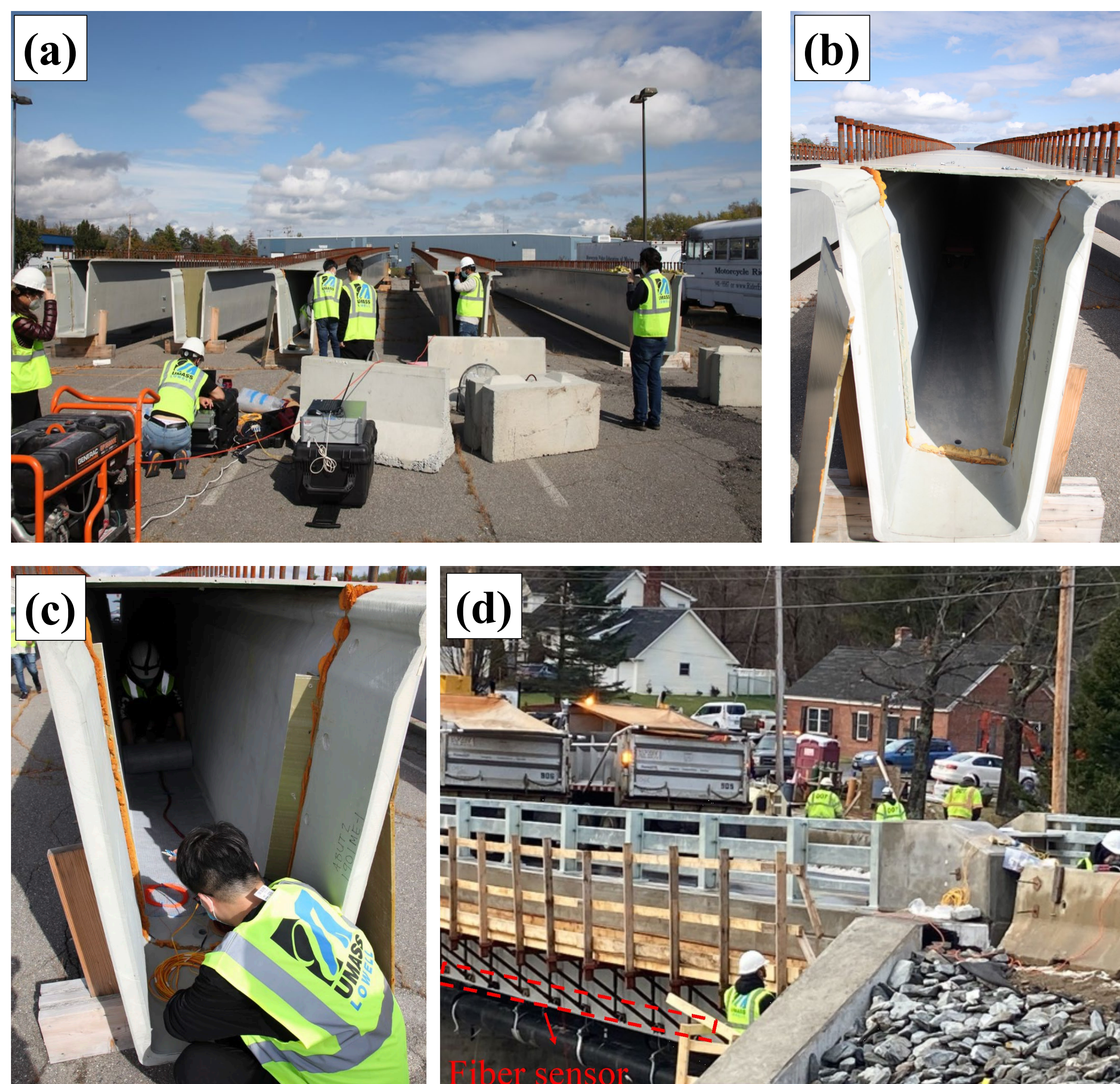
Fig. 3 Pictures of installation. (a) UML team working on the girders. (b) Side view of the bridge girder. (c) Installing fiber connectors. (d) Picture of the bridge and the location of fiber sensing textile.
